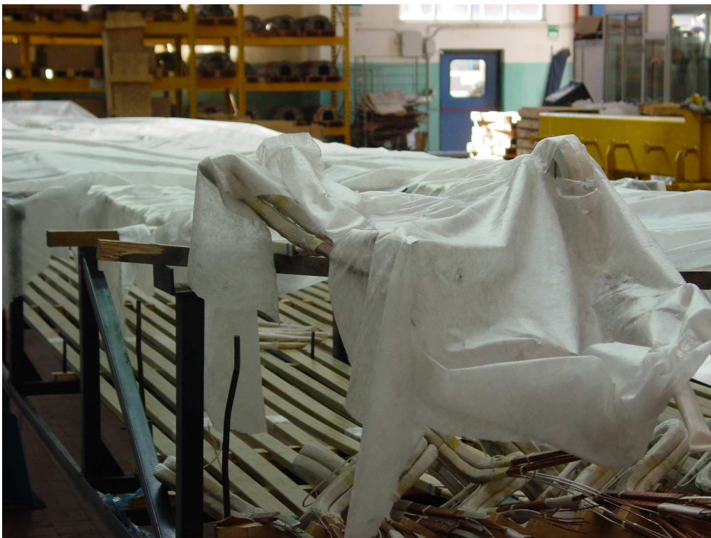
Fig. 12: Bus-bars without nylon bags on the rack
