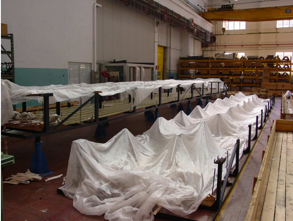
Fig. 11: Bus-bars rack on supports
