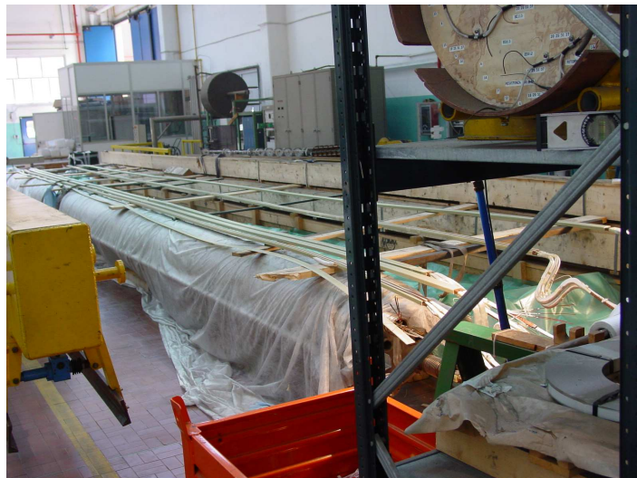
Fig. 5: Bus-bar ends under lamps
