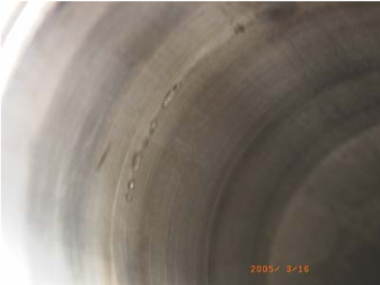
Figure 6 : Root concavity – Defect N°515
