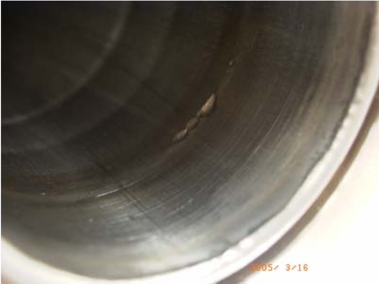
Figure 7 : Root concavity – Defect N°515
