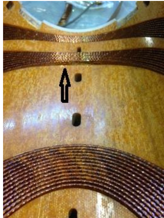
Fig. 39: Cable protruding inside the aperture in the coil heads of MBXFS1 (see black arrow)
